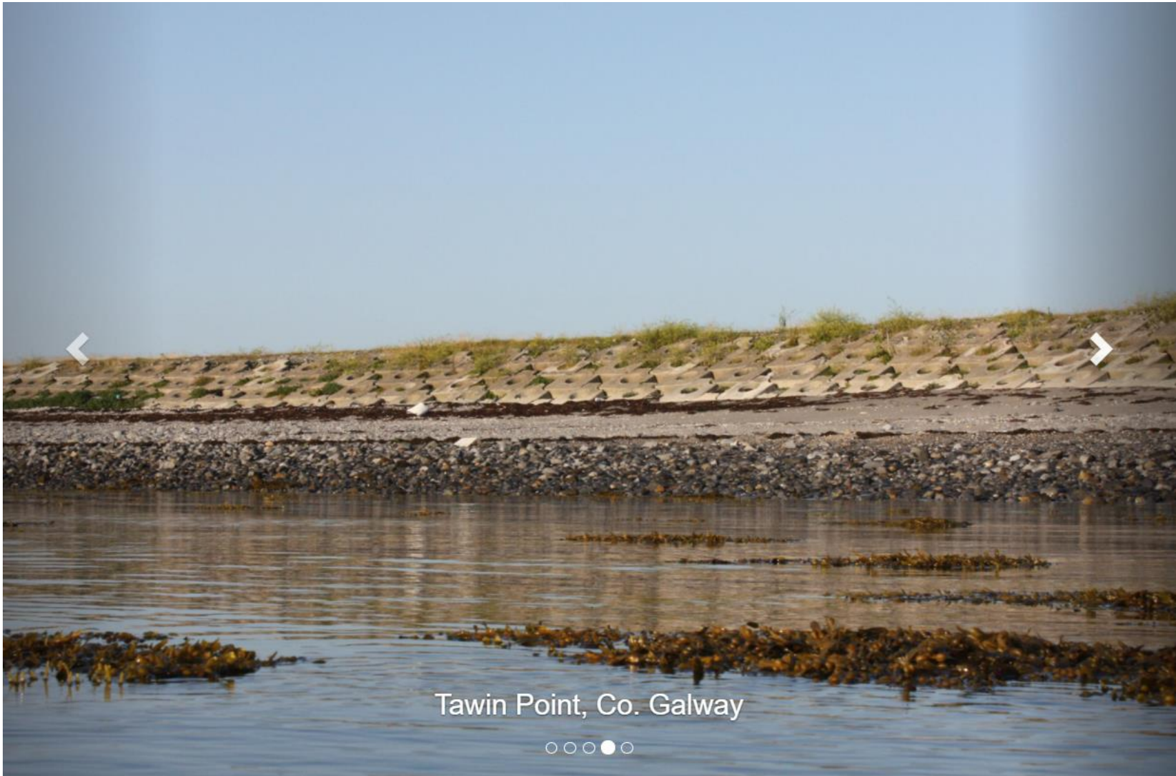
Plate 2. View of interlocking concrete block revetment at Lurgan Island (extract from ECPS Ltd. Ecab.ie).
