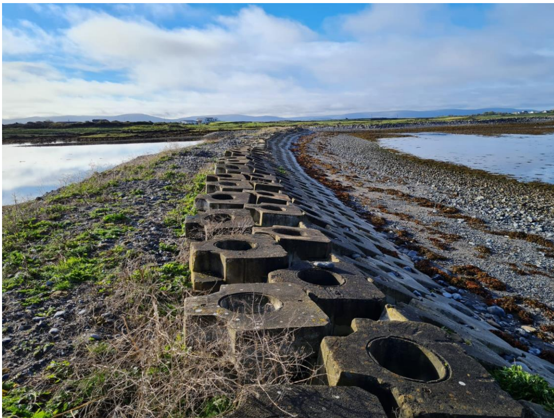
Figure 7-4: Flattening out of top layer of sea defence blocks, Lurgan Island, October 2021.
