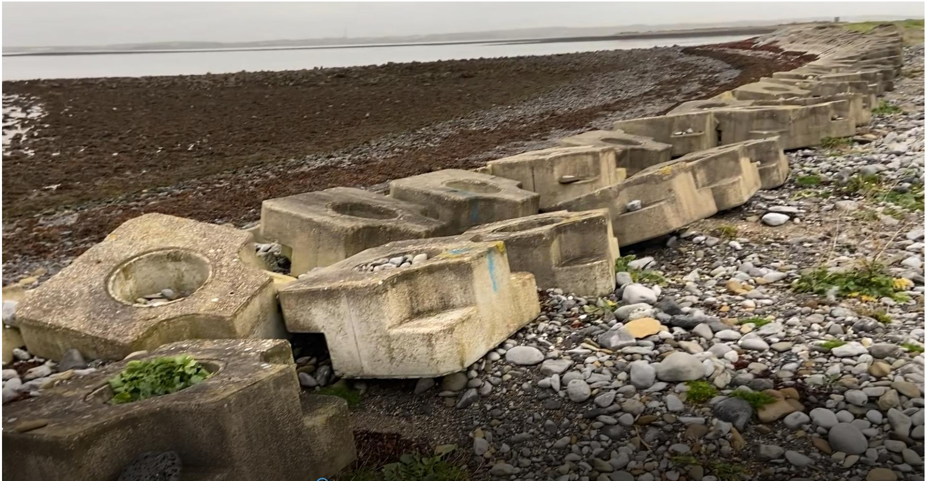
Plate 4. Lowered and displaced section of ECAD revetment at Lurgan Island (November 2021).
