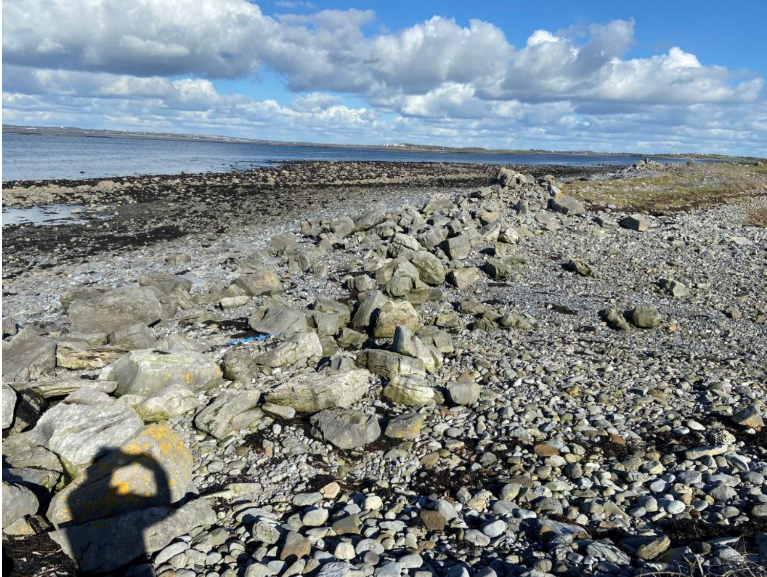
Plate 6. Significant site of bank erosion 600m to the east of the subject lands where rock armour protection had been placed previously (late 90's) but has been undermined and significantly lowered forming ineffective protection.
