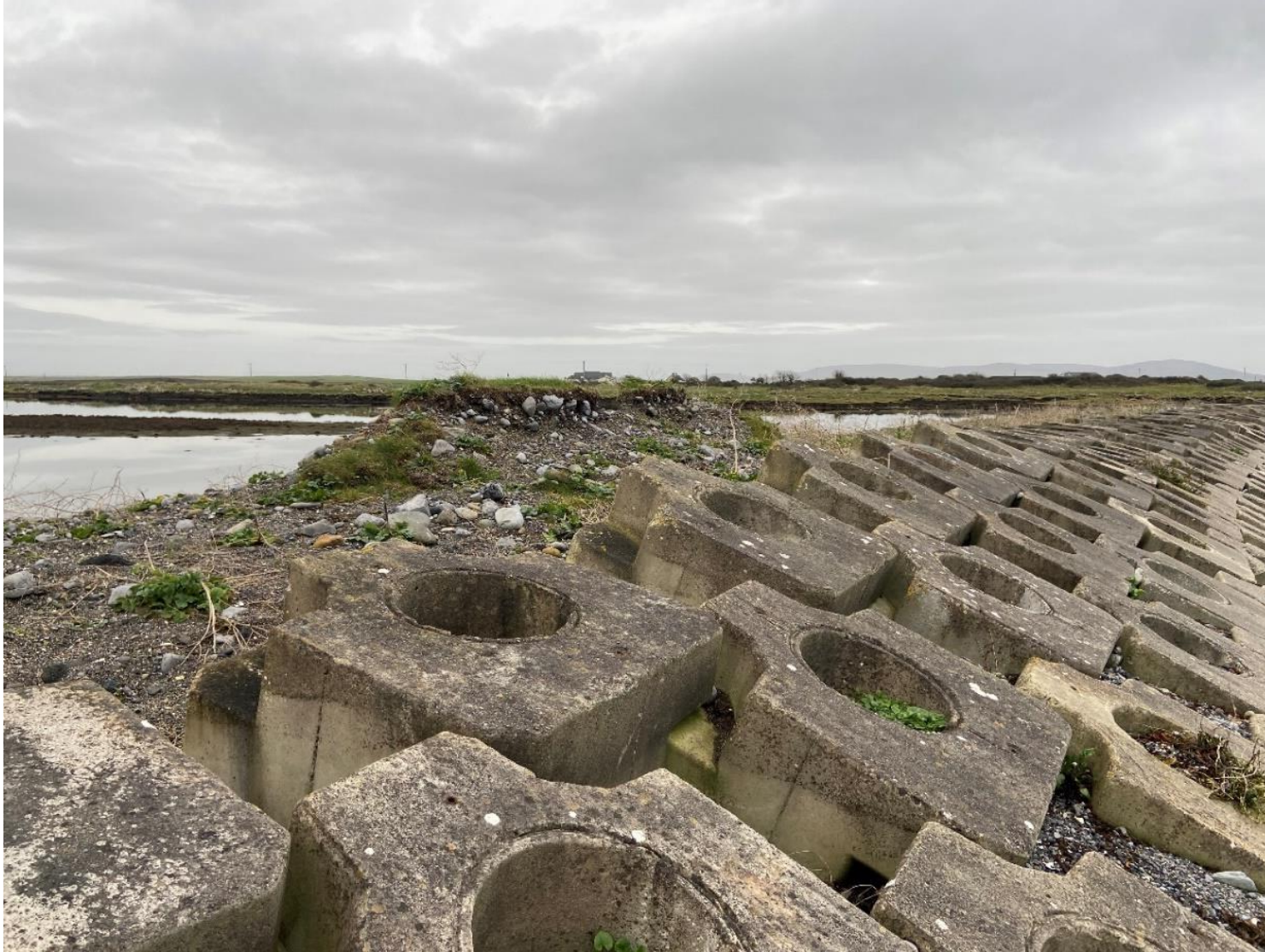
Plate 5. Photos of revetment taken in November 2021 showing substantial undermining of the revetment armour blocks and erosion of the headland behind the defences.
