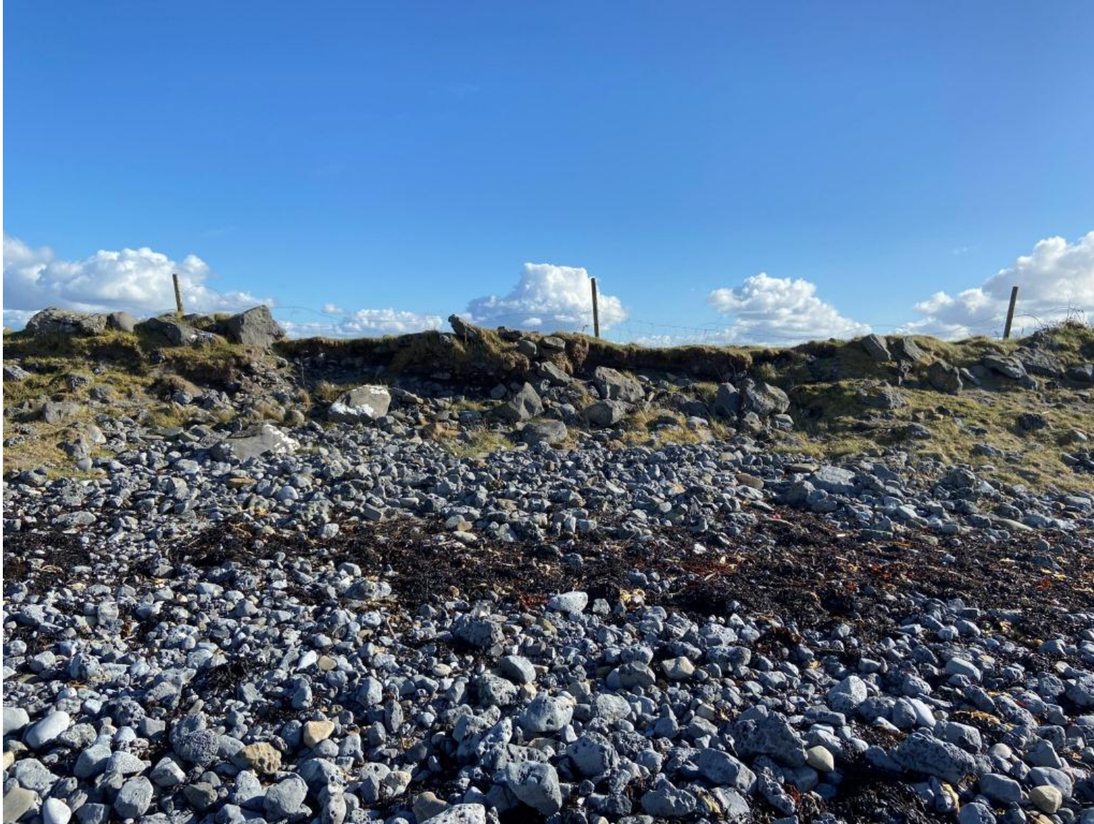
Plate 7. Significant local Bank Erosion 80m west of the subject lands.
