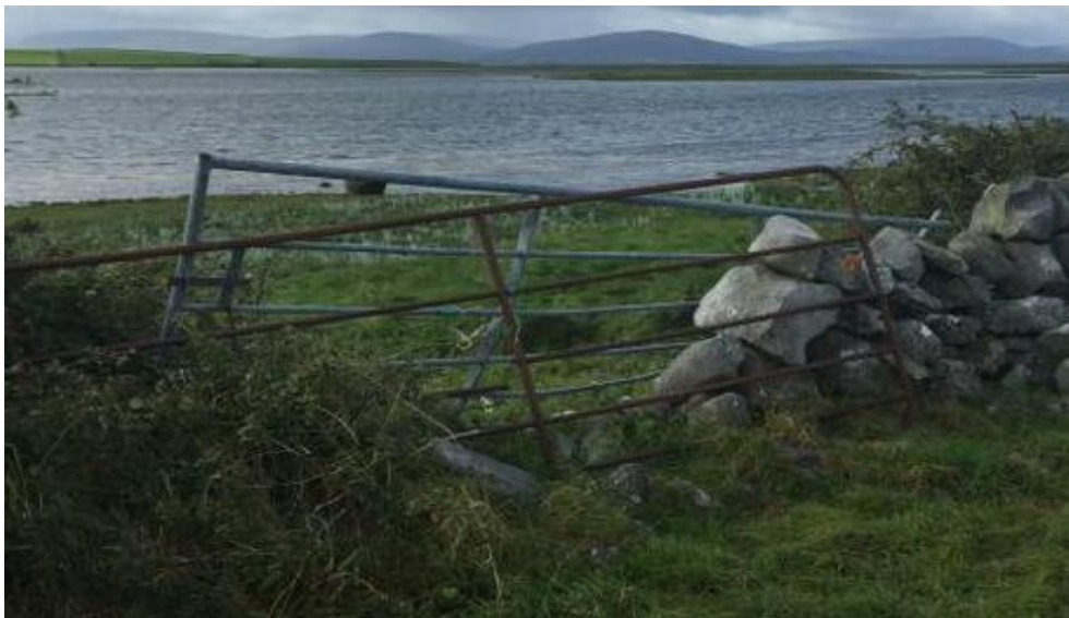
Figure 4-6: Gates in need of repair.
