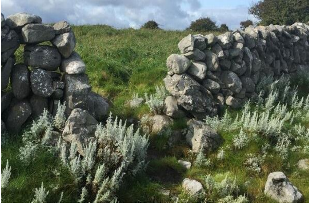
Figure 4-5: Collapsed stone wall that requires rebuilding.
